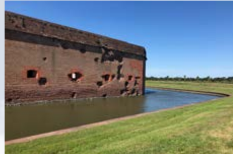
Cannonball Holes in Ft. Pulaski’s Brick Walls
