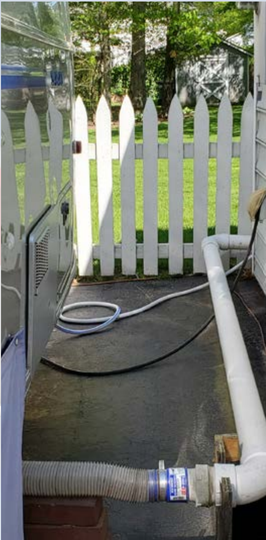
Full hook-ups are installed on the side of the Brodsky home. They enable the Airstream to accommodate overnight guests in comfort.
