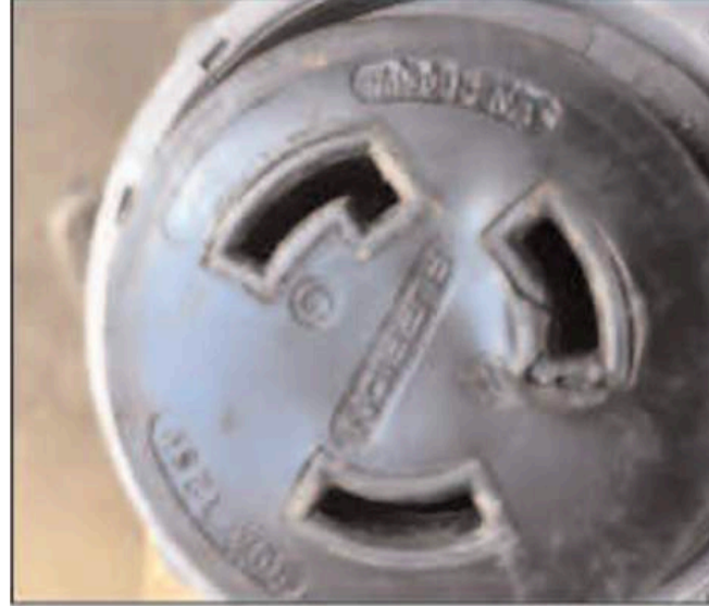
Evidence the shore power plug got very hot.
