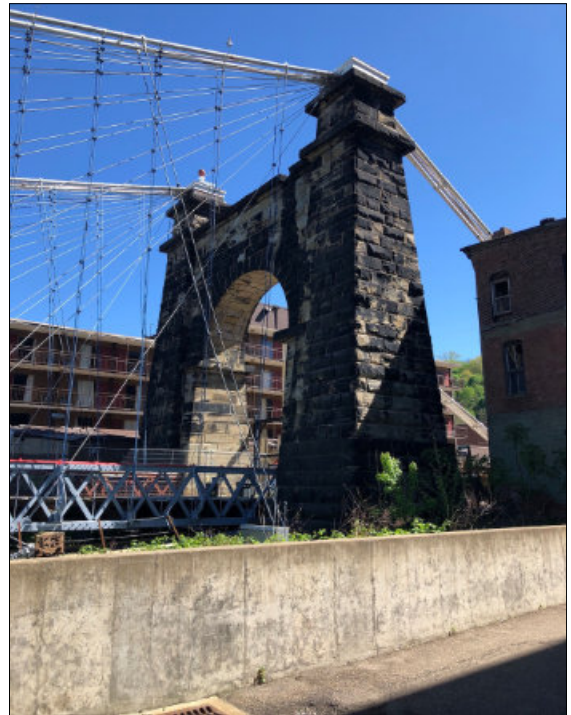
The Wheeling, WV suspension bridge, completed in 1849, could have been used by Civil War troops, currently under renovation.
