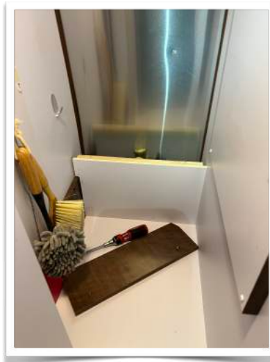
Inside the back of the closet, I removed the top panel but getting tools in there to replace the part was a challenge.
