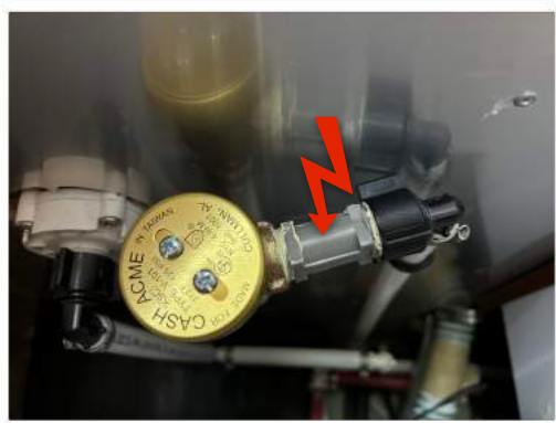
Check valve attached at both ends viewed from above
